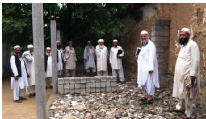
A view of class room being constructed through community contribution at MSB 021-(Manshera)
