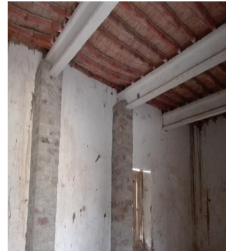
A view of newly replaced ceiling of class room at PSC-189 Doaba, Thall
